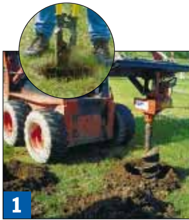
1 Deep footings or tough soil make hole-digging a job for a power auger. For easier sites and for final cleanout, you can use a manual posthole digger.
