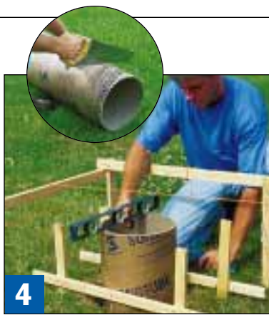
4 Use stakes and crossbars to suspend the footing forms about a foot off the bottom of the hole. Drive 1 1/4” screws to hold the form level in one direction.
