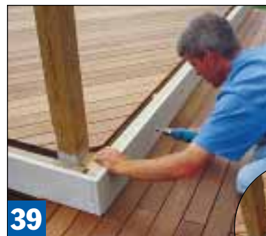
A 1x8 fascia, stained to match the house siding, covers the subfascia before the ribbon boards go on.
