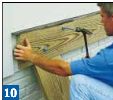
10 If possible, drill through the rim joist of the house frame, then bolt through the ledger and rim joist. Or drive lag screws, but be sure you hit that joist.
