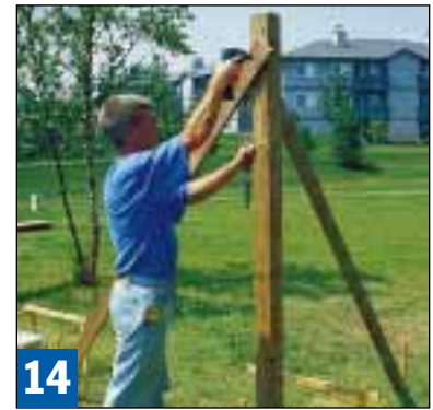
14 Tie temporary braces to wood stakes and to the top end of each post, so the post alignment is kept intact.
