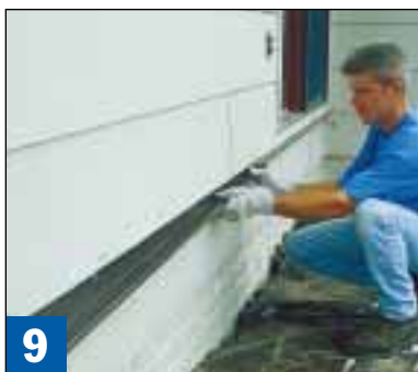
9 Whether or not you remove the siding behind the ledger, tuck metal flashing under the siding course above it to divert water away from that area.
