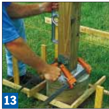
13 Center the post in its bracket, check it for plumb, and use a pair of clamps to hold it in place until it's bolted.
