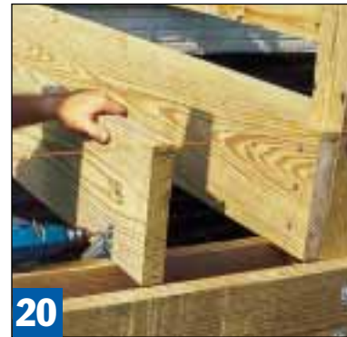
20 With a string line to keep the ends of the field joists aligned, fasten them to the hurricane ties and joist hangers.
