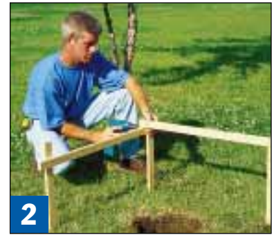
2 Assemble batter boards just outside the deck layout. These let you place and adjust string lines to mark the post locations precisely.
