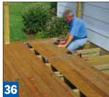
Work your way toward the house one section at a time. Later, you can go back and fill in the open courses.
