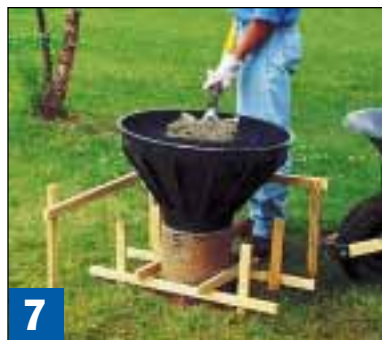
7 An inverted BigFoot footing form saw duty as a funnel for our concrete pour. Use care not to disturb the cardboard forms or you'll dislodge their screws.
