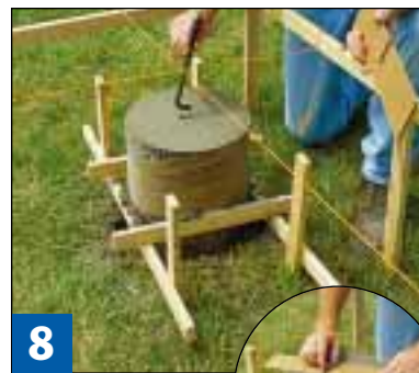
8 Use the strings to guide the anchor bolt placement, then slide a "keeper" board under the nut.
