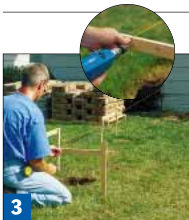
3 Tie strings close to their final location and check for square corners (see Skill-BUILDER). Drive screws to mark the centers and edges of the posts.
