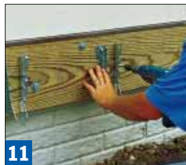
11 Metal hanger brackets will support the deck joists at the ledger. Nails don't hold as well and tend to squeak after a while, so use screws to fasten these.
